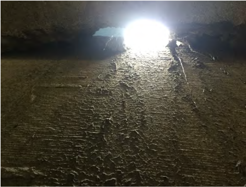
Damage to downstream left bank panel 1
